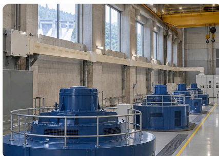
Power generation plants
