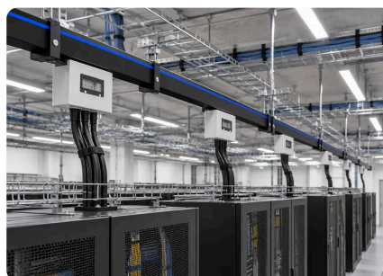
Telecom central offices
